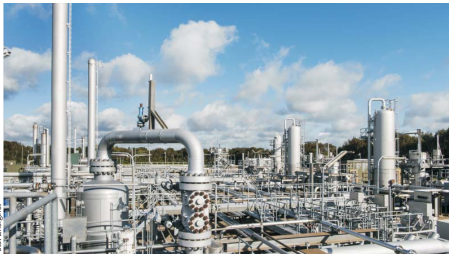
Gas Storage Danmarks gaslager i Stenlille.
