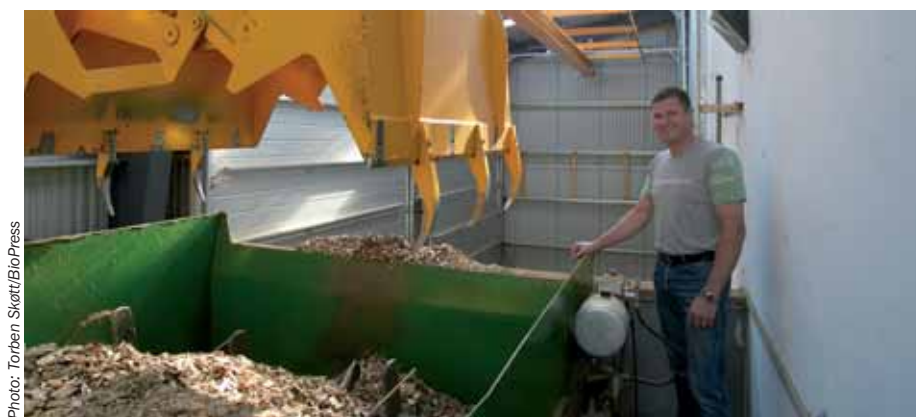
Production manager Torben Brand Andersen at the crane, which supplies wood chips to the vaporizer and the boiler.
