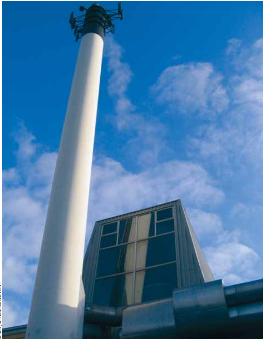
The district heating plant in Øster Toreby, where they have installed a condensation system for the largest of the two straw-burning boilers.
