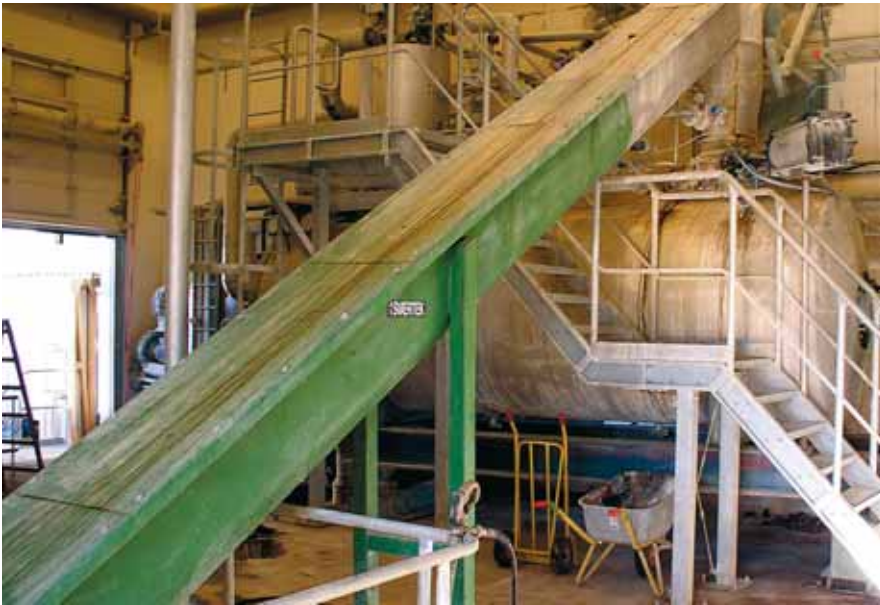
Autoclave plant at GreenFarmEnergy in Over Løjstrup. Here the biomass was pressure-cooked at a temperature of 147°C for half an hour to an hour, and 4-7 per cent burned lime were added.
