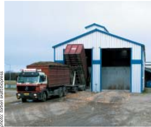
The heat and power plant in Harboøre, which is based on the gasification of wood chips, has the largest number of operating hours of any gasification plant in the world.
