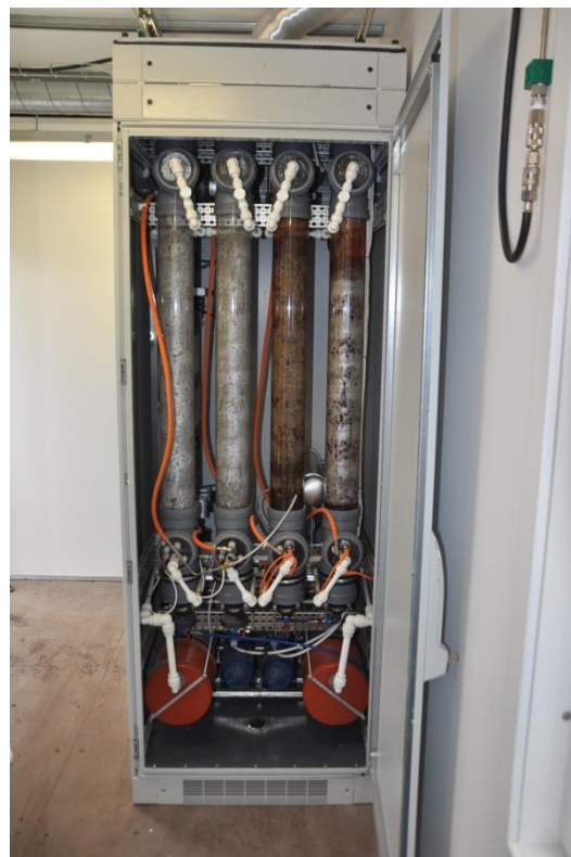
Picture 1 Cleaning unit.
